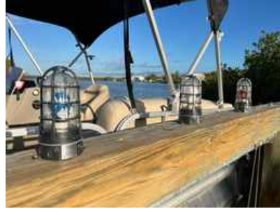
Dock guidance lights (switch is to the right of the lift)
